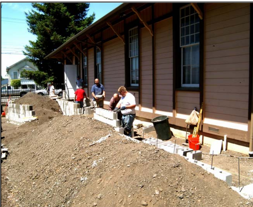
The crew working on the second segment of wall, behind the SLHRS former S.P.
