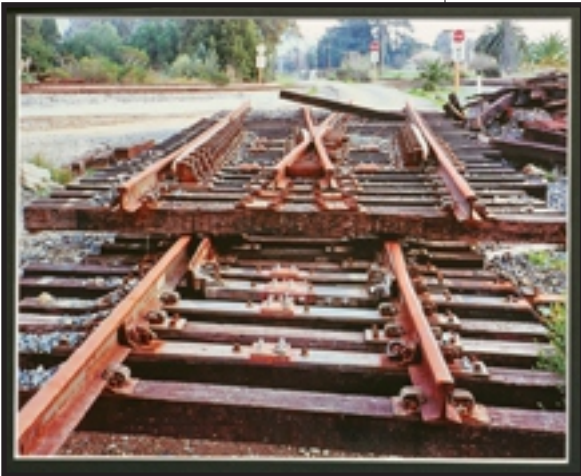
Photograph - Tracks & structures - 1 st place - Eugene Brichacek - sring switch ready for install
