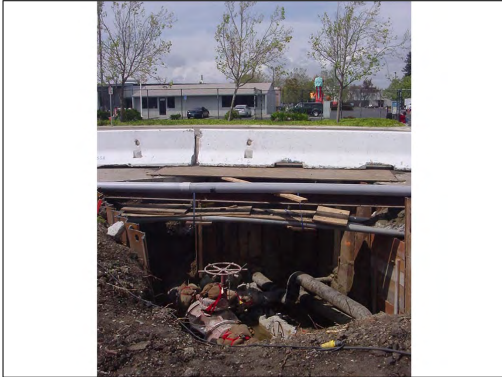
Underneath Winton Avenue in Hayward. Puts a slightly different perspective on it.
