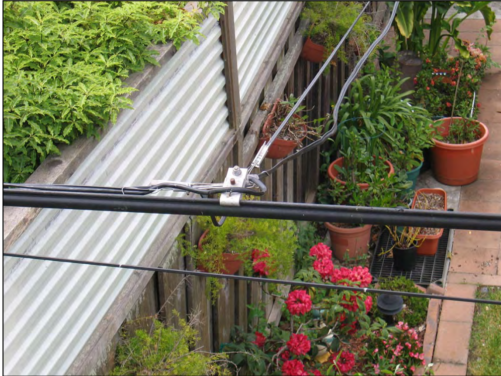
This is a close up of how the cable and phone lines travel to get to the houses. The taught one is phone. The one of questionable neatness is the cable.
