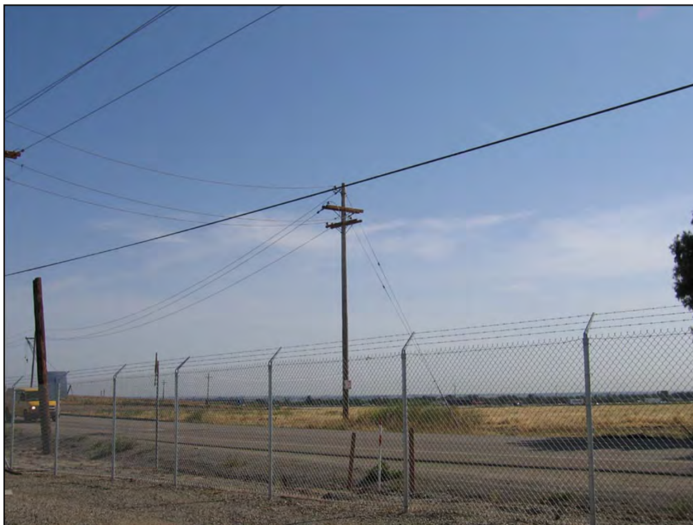
Another Power pole
