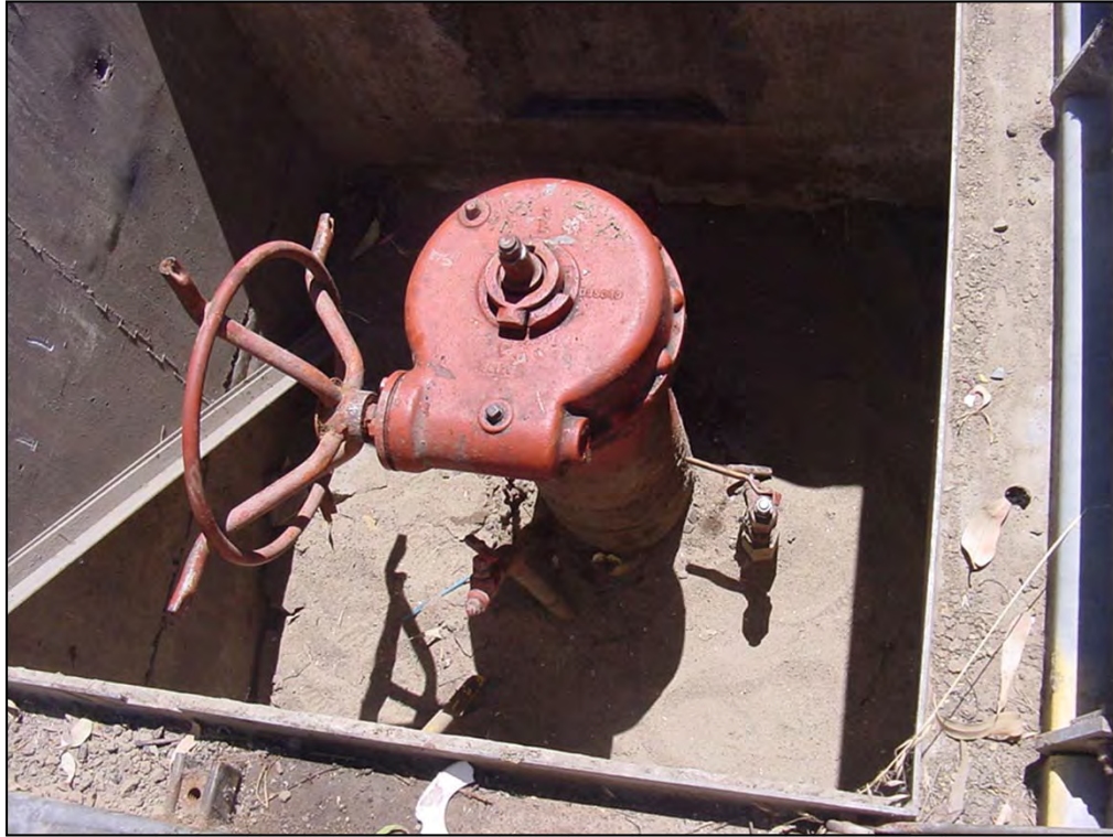
Or the topworks to a 30 inch valve.
