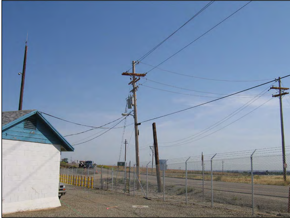
Connected to a joint pole
