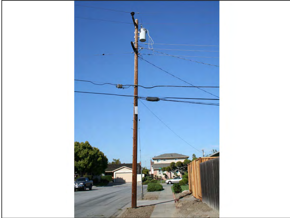
Here is your typical city street joint pole. Notice the primary on top, the secondary, the cable TV, and then the telephone.
