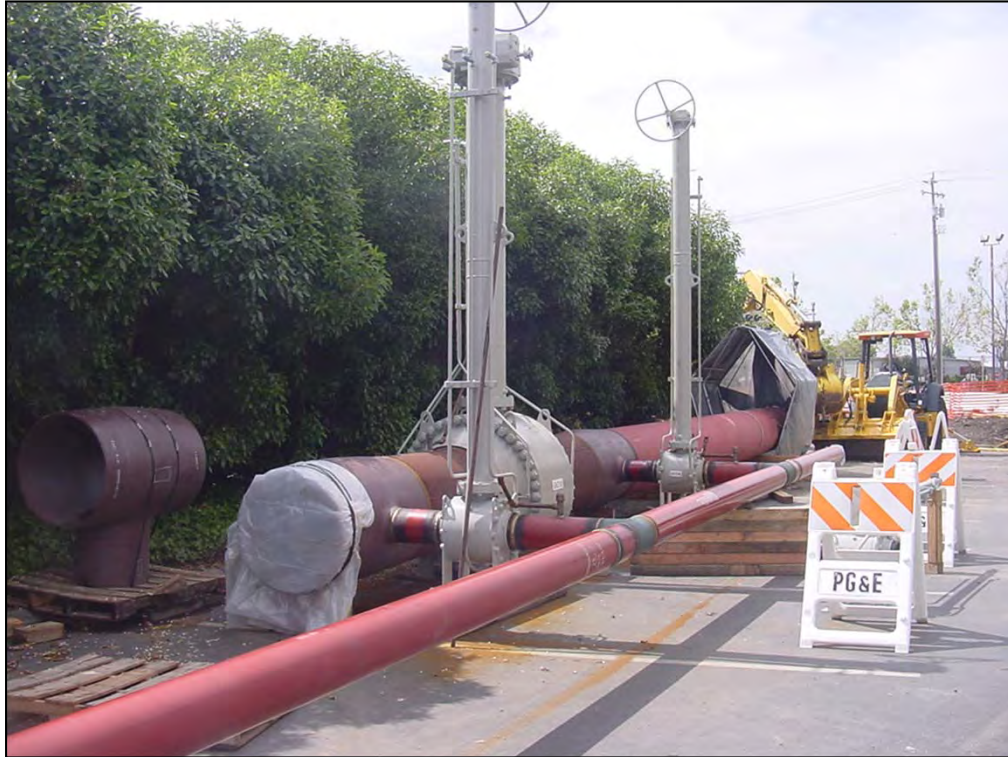
This is the new valve set we replaced that old valve set with.
